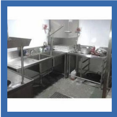
Dish Washing Equipment
