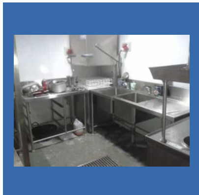
Dish Wash Equipment
